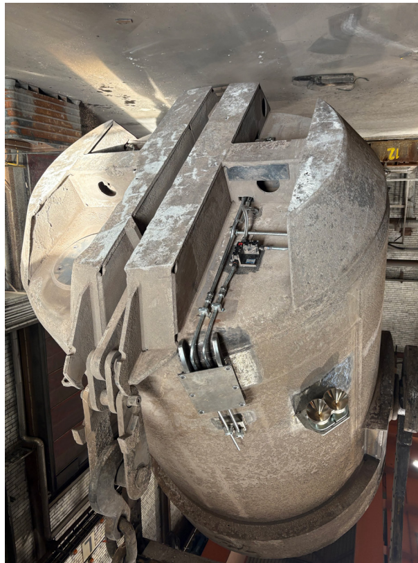
Image 3: Newly Installed Feeding Lines for a Two-Porous-Plug Application.
